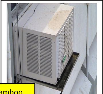
Air condition trays
