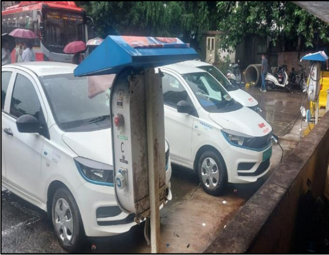
Electric charging station
