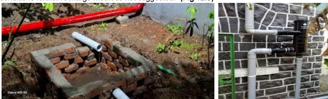
Fig 12.9: Rain water harvesting structure in campus
