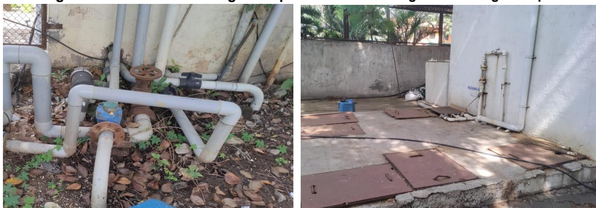
Fig 12.6: Ismail Yusuf College Campus: Municipal water supply & underground storage tank
