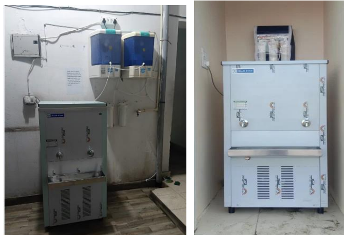
Fig 12.2: Ismail Yusuf College Campus: Water Filter plant in Campus
